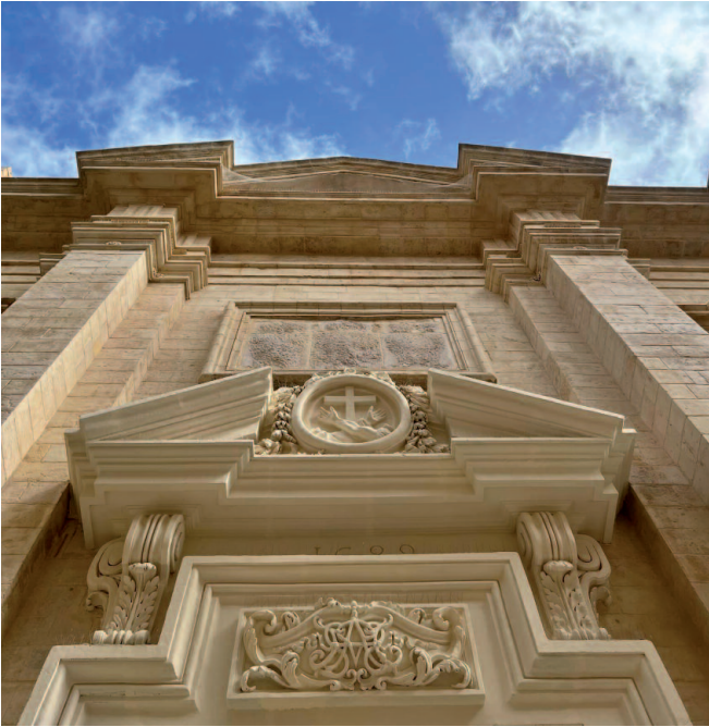
Fig. 2. Detail of the façade of the Church of St. Mary of Jesus (Ta' Giezu) in Valletta designed by Médéric Blondel in 1687.
